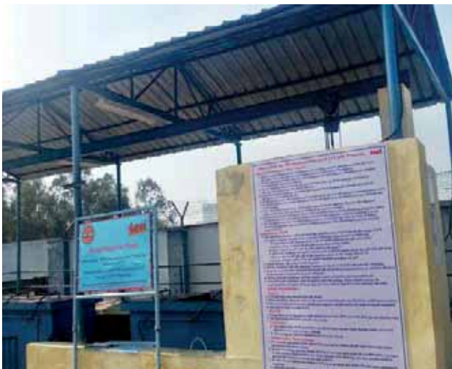
A TEAM plant at Neptha Cracker Unit, IOCL, Panipat, Haryana
